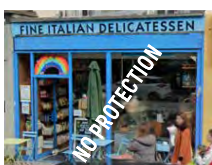
46 Cross St, cornice, brackets Aluminium, needs rebuild
