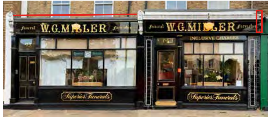
93 Essex Rd, Cornice missing 95 Essex Rd, Bracket missing
