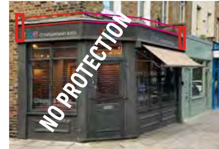
52 Cross Street, Cornice and Brackets missing, mirror other end 40 Cross
