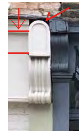
47 / 49 Cross St, Cornice too high bad gap details, should be lower align to bracket.
