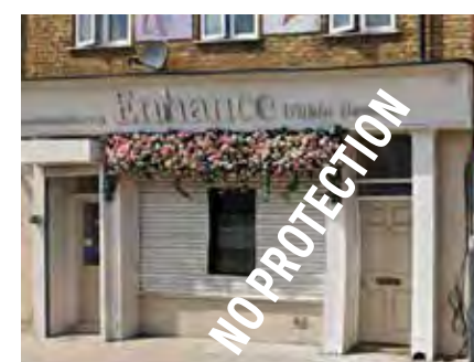
61 Essex Road, roller shutter sign obstructs cornice fascia
