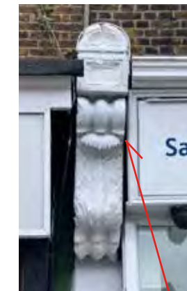
70 Essex Rd, bad gaps
