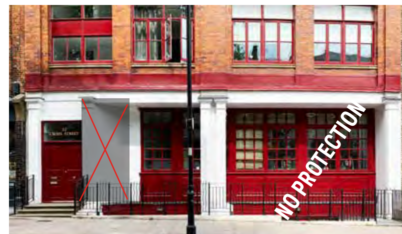
30 Cross St, Changes in X area. Paint red to match windows
