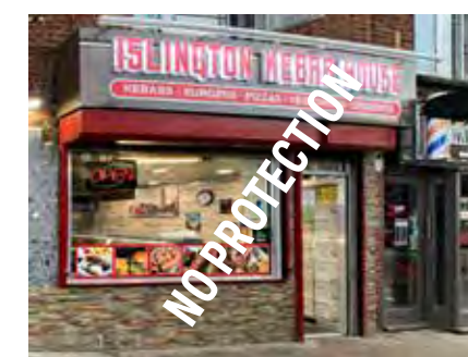
63 Essex Road, roller shutter sign obstructs cornice fascia
