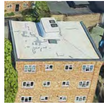
Modern Membrane Flat roofs.
