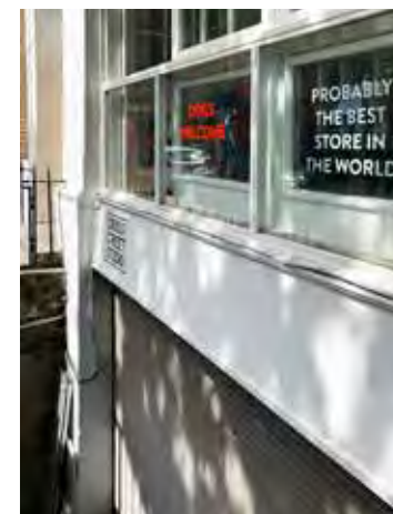
26 Cross St, Harmed Roller Shutter basement
