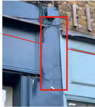
4/2 Shillingford St, missing Console Bracket
