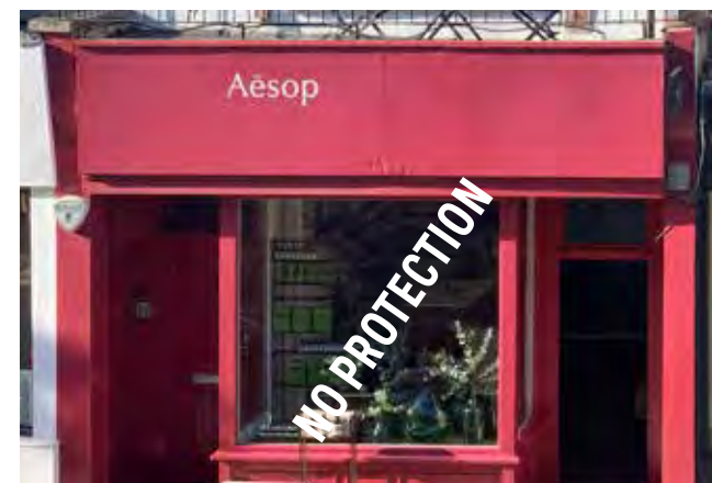
56 Cross Street, Damaged Console Bracket, No Cornice, Signage Fascia too large, Out of Scale.
