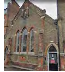
12 Fowler Street secondary glazing
