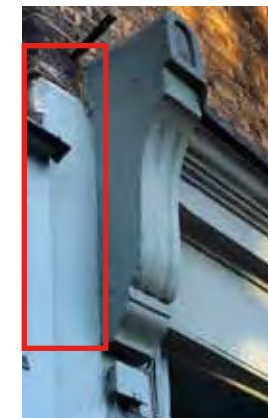
38 Cross Street, left Console Bracket missing
