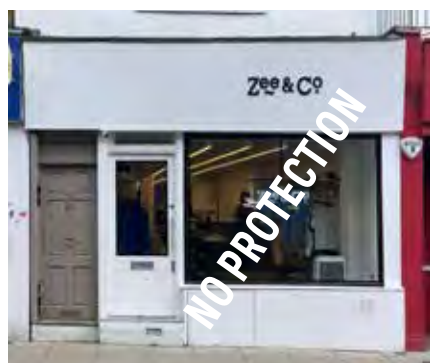
58 Cross St, Fascia Oversize missing Cornice and Brackets
