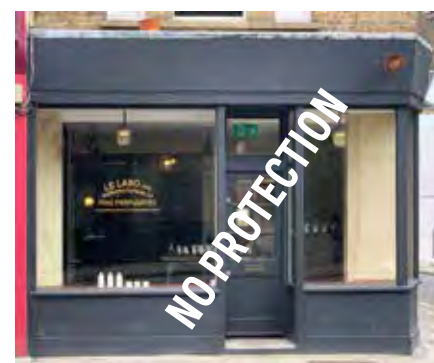
54 Cross St, Fascia Oversize missing Cornice and Brackets
