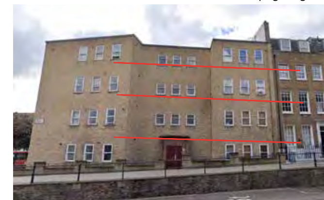
1-8 Belmont House, Cross Street Poor windows, details, and facade composition out of alignment with Heritage Terrace. Suitable for external insulation, new windows, and facade details.
