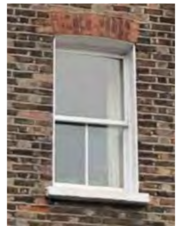
Cross Street- Harmed sash on listed Georgian
