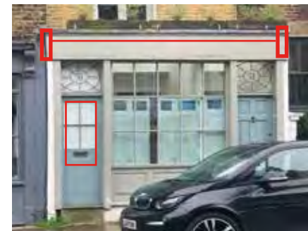
51 Cross Street, Now a House, Cornice and Brackets missing door window to match
