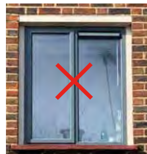
Nearby Florence Street same building above, replaced vinyl window
