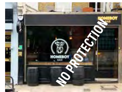
108 Essex Road, missing cornice and right bracket
