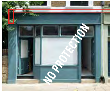
8 Shillingford Rd, Cornice and Brackets missing
