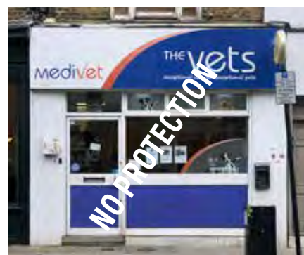
60 Cross St, Signage oversize Aluminium needs rebuild
