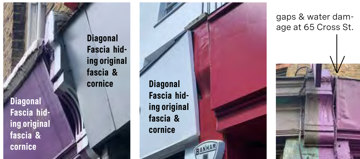
65/67 Cross Street, Signage Fascia large, obstructs bracket
