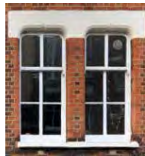
Distinctive Victorian 36/34 Cross Street wide glazing bars which could take sealed double glazed units mounted into this original timber sash, or see page 88 vacuum glass.
