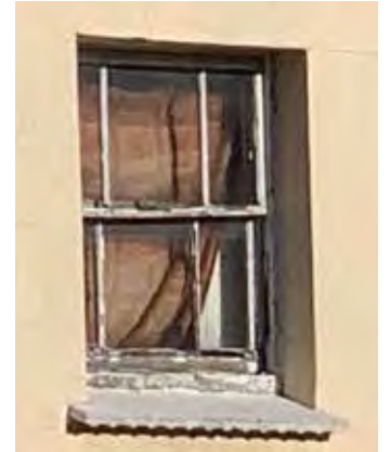
Cross Street- rotten, double glazed required
