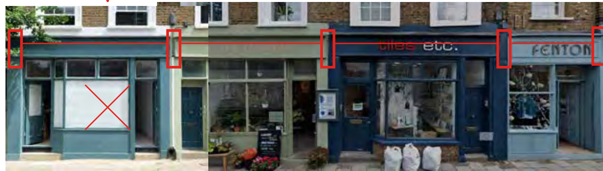
8, 6, 4 and 2 Shillingford St, Heritage damage allowed no Console Brackets or Cornice.
