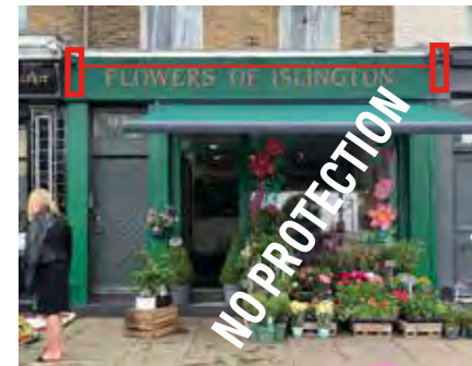
97 Essex Rd, Cornice and Brackets missing
