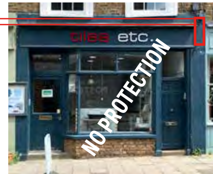
4 Shillingford Rd, Cornice and Brackets missing
