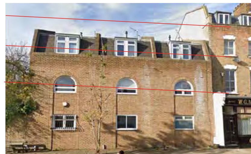
87, 89, 91 Essex Road Out of scale, poor windows and facade, floor heights not matching original terrace. Suitable for external insulation, new windows, and additional storey.
