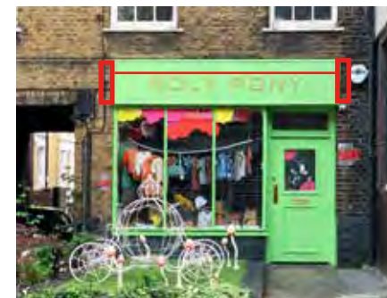
41 Cross Street, Cornice and Brackets missing
