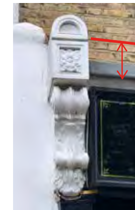
93 Essex Road, cornice missing
