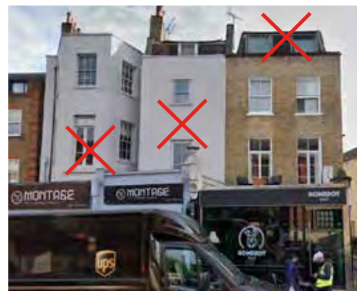
112, 110, 108 Essex Road Shopfronts harmed, new windows mismatched with reduced size. Suitable for external insulation & windows.
