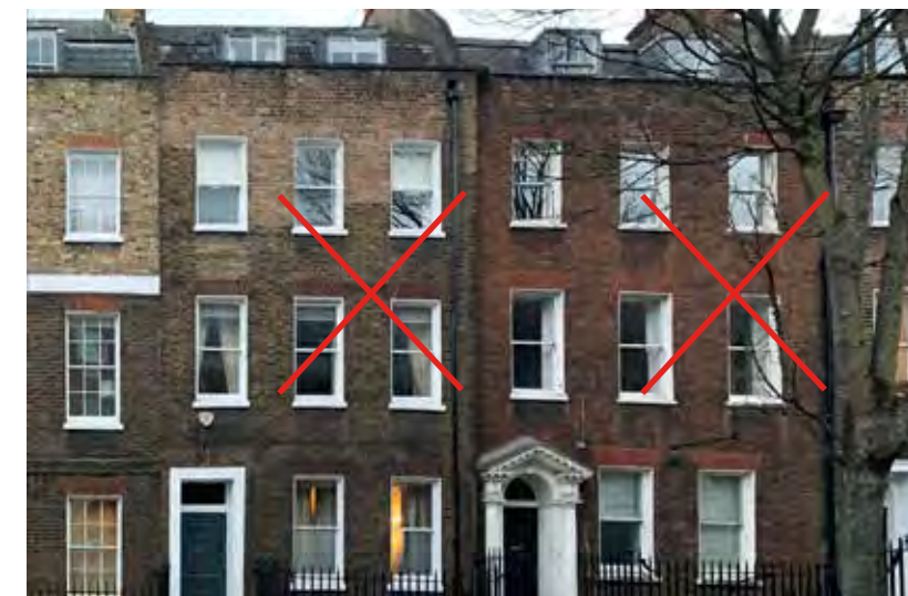
Harmed 1 over 1 windows should be replaced with sympathetic historic pattern 6 over 6 double glazed, Cross Street Listed terrace
