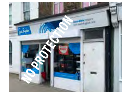
72 Essex Road, roller shutters sign obstructs cornice fascia
