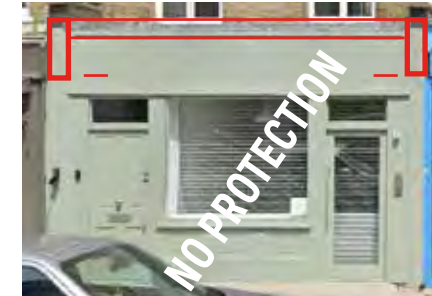
50 Cross Street, Cornice and Brackets missing, low fascia
