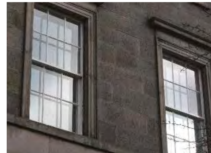
Secondary window visual impact of reflections on inner secondary windows harms heritage in Conservation Area. Research found by the trial installation of different double glazed unit types in Edinburgh Georgian tenements, by the Changeworks project mentioned above. 2
