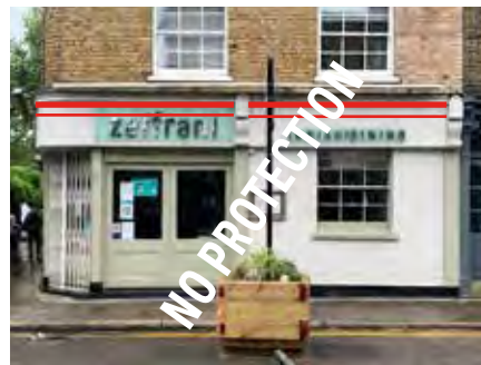
47 Cross Street, Fascia sign not separate letters, bad flashing with Cornice missing
