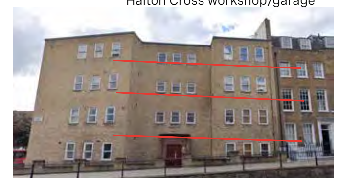
1-8 Belmont House, Cross Street Poor windows, details, and facade composition out of alignment with Heritage Terrace. Suitable for external insulation, and facade details.
