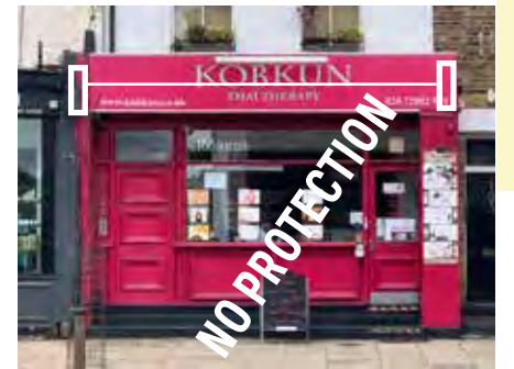
101 Essex Rd, Cornice and Brackets missing
