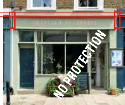
6 Shillingford Rd, Cornice and Brackets missing
